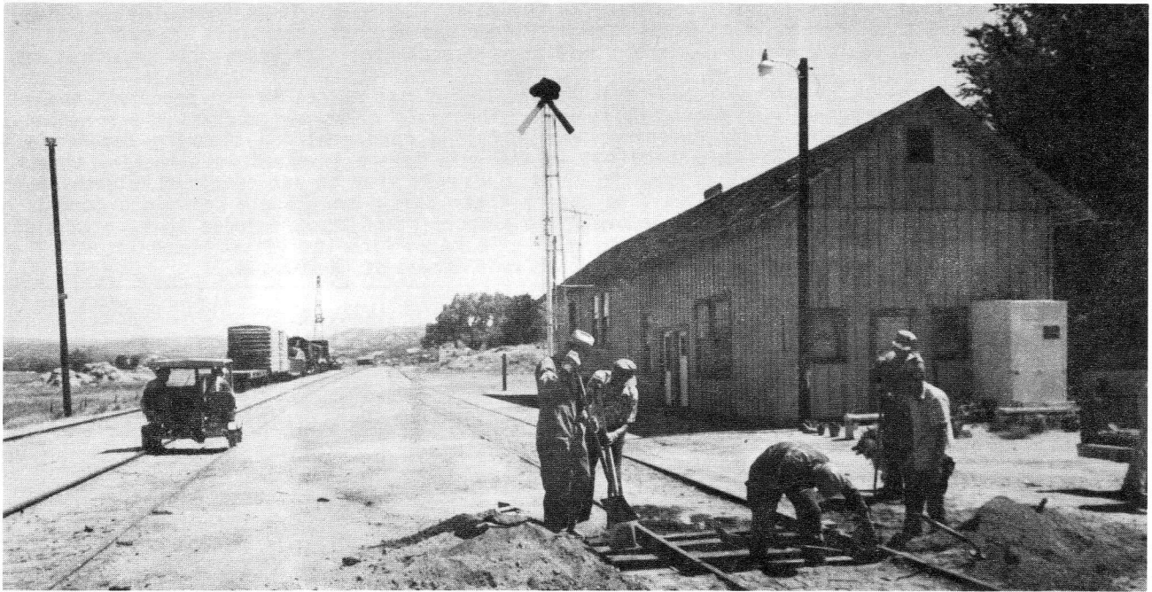
Trackwork on our SD&A is a never ending chore. The house track at the Campo Depot is a prime candidate for new ties. Shown here digging in new wood are (from left) Norm Heil, Gaylen Dyreng, Craig Coney, Geoff Shepherd and Floyd Lake . Other SD&A trackies have been Jim Lundquist, Charles Alban and Larry Rose . At left the fire speeder waits for the morning train to roll out of the museum grounds. (L. Rose photo)
